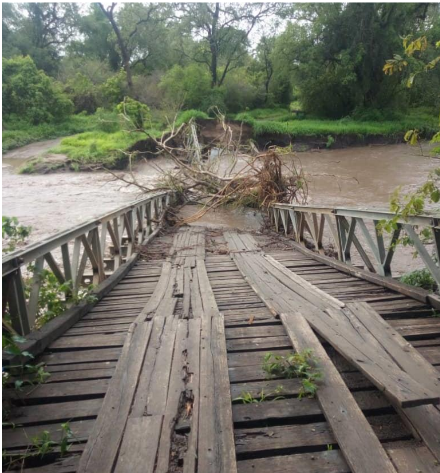
Figure 38: Entrance Bridge at Lengwe NP that collapsed in January 2020 due to flooding of Mkombezi.
