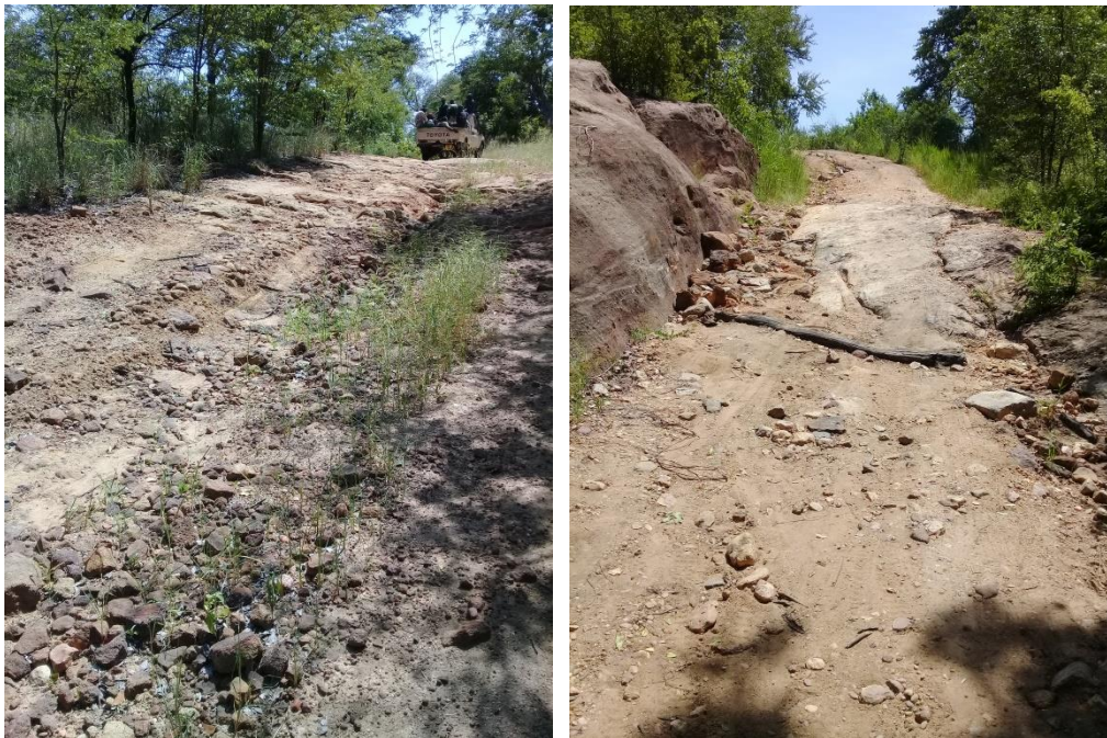
Figure 13: Poor Road conditions and network
